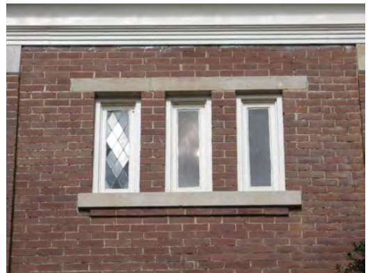
Unpainted masonry walls shall be left unpainted unless the brick is badly damaged or has numerous repairs (First Presbyterian Church, 300 Tennessee Street).
