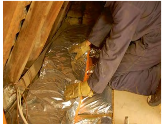
Adding attic insulation is often the most important method to insulate historic buildings and save on energy costs.
