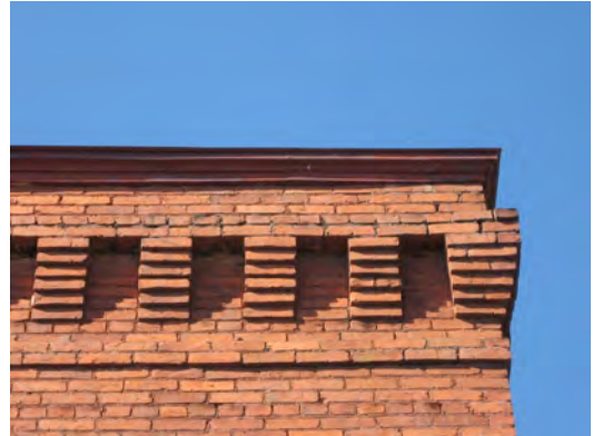
Stepped or “corbelled” brick courses were used to decorate several buildings in the downtown area such as at 45-55 Court Street.
