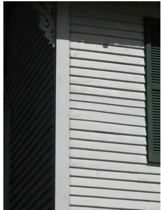
Preserve and maintain original wood siding through proper painting and regular maintenance (140 College Street).
