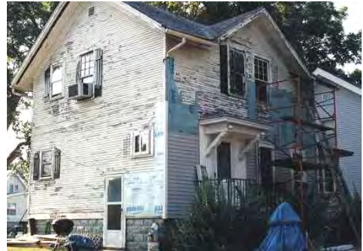
The application of vinyl siding often involves the removal of original historic features and can cause condensation in the walls.
