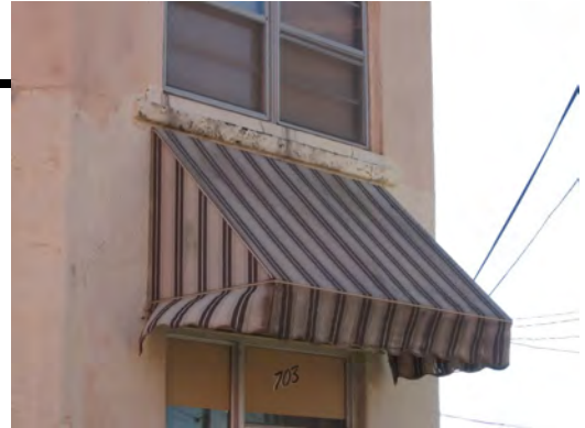
Awnings are appropriate for commercial storefronts and entrances such as at 39 Court Street.
