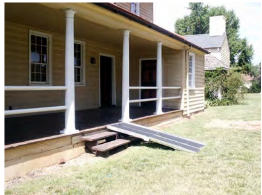
Consider the use of temporary or portable ramps rather than more permanent wood or metal ramps.
