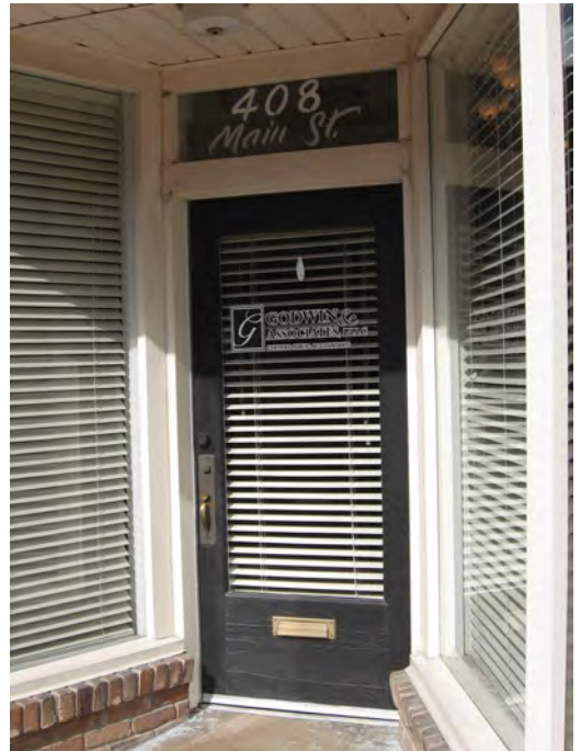
This entrance features a large transom as well as an original single-light glass and wood door (408 Main Street).
