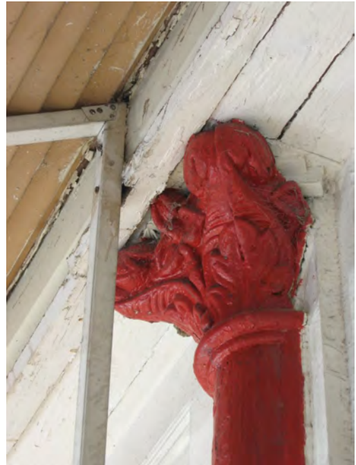
Cast iron was a popular feature on commercial buildings of the late 19th century, as seen at 242 Guinn Street. This cast iron was produced by the Mesker Company of St. Louis and there may be other cast iron features hidden beneath added storefront materials in the downtown area.
