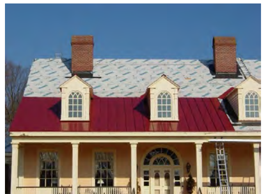
New metal roofs shall match historic profiles of crimping and spacing to match original metal roof designs of the dwelling's period.
