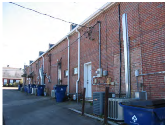
Install HVAC units and store garbage receptacles behind commercial buildings, as in the 400 block of Main Street.
