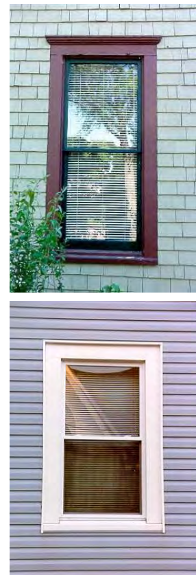
Replacing historic windows with vinyl windows is neither cost effective or compatible with a building’s historic character.
