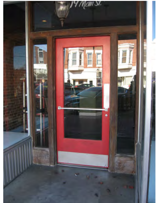
The building at 409 Main Street has an original historic wood door and wood surround with sidelights and transom.
