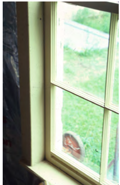
If replacement windows are necessary they shall have divided lights as shown above rather than applied muntin bars.
