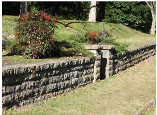
It is important to preserve and maintain original retaining walls of stone, brick or rock-faced concrete block such as this wall at 155 Williams Street.
