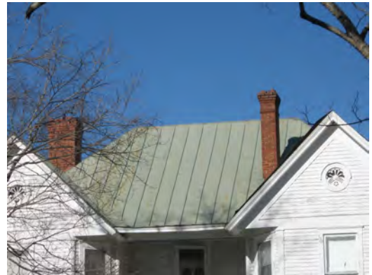
The dwelling at 130 College Street retains its original metal standing seam roof—these types of roofs should be repaired and retained.
