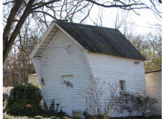
Historic wood frame outbuildings such as at 215 Church Street remain extant and are important resources of the property.
