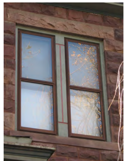
Storm windows are recommended to conserve energy.
