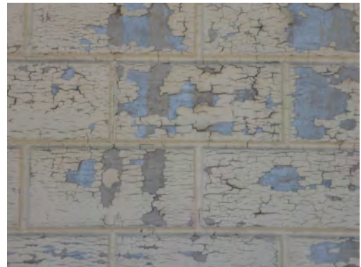
Minor work would include the removal of original paint and repainting (470 Water Street).
