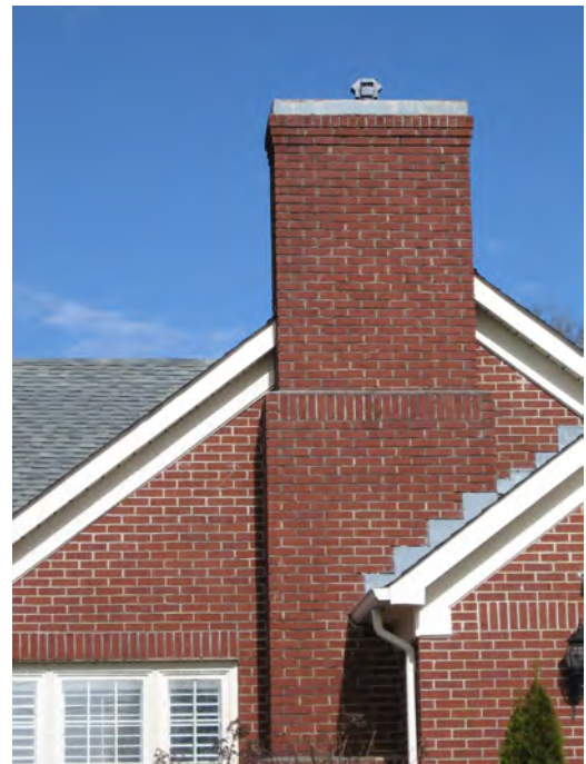
Keep masonry surfaces such as exterior walls and chimneys in good repair (250 College Street).
