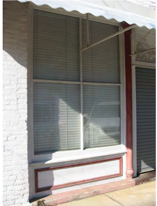
This original storefront at 242 Guinn Street retains its frame bulkhead, four-light display window, transom and cast iron column.
