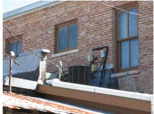
Heating and cooling units shall be sited at rooftops where they are not visible from the street (above) or are screened through landscaping or fencing (below).
