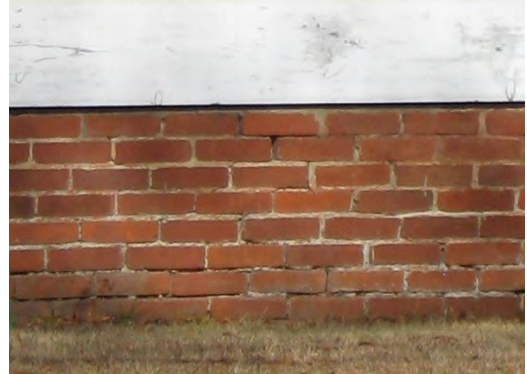
Brick foundations shall be repointed with brick and mortar to match the original.
